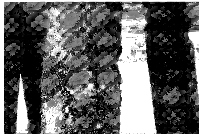
Pile badly damaged due to collision with a barge
