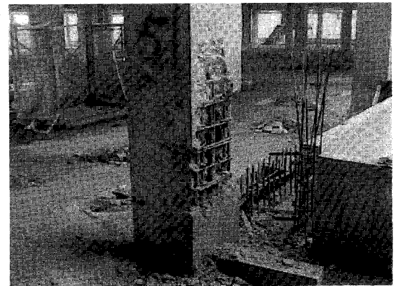
Figure 3 : The removal of honeycombs in a defective concrete column due to bad concreting practice at site
