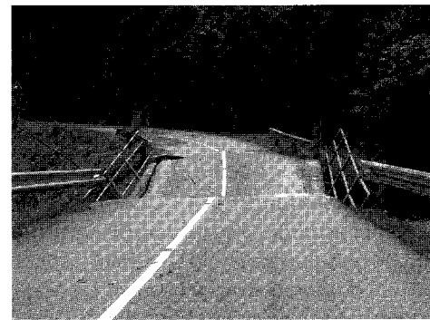
A collapsed single span steel buckle plate bridge structure due to scouring of abutment
